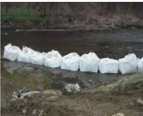
Giant sandbags were placed by the front-end loader to divert stream flow away from disturbed areas. This erosion and sediment control was purchased from ACF Environmental.
