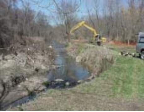
This photo shows the existing conditions of the eroded bank and gravel bar.
