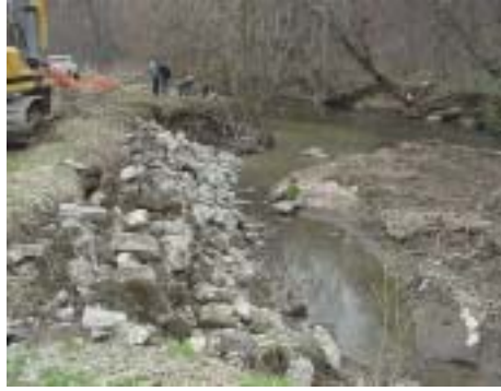
The filling of the eroded bank began with covering an exposed sewer line with several tons of R-5 stone. The R-5 was then covered with material from the gravel bar.
