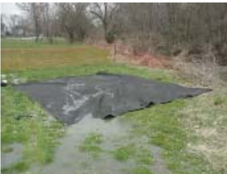
Water that passed under the sand bags was pumped into a filter bag away from the disturbed section. The filter bag drained away from the bank preventing any trenches from forming.
