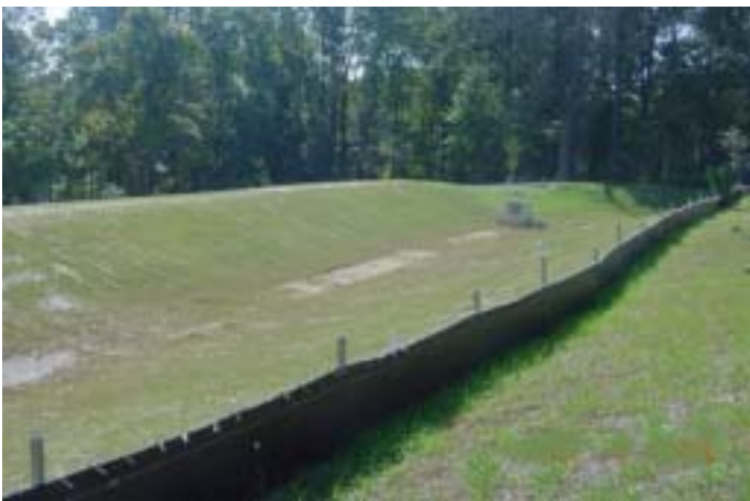
The basin is designed to infiltrate runoff from a ten-year storm.
