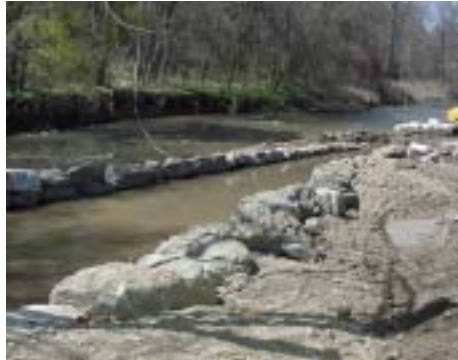
The W-weir was constructed one arm at a time. Here you can see the first arm nearing completion. Once completed, the sandbags were switched to the other side of the stream and the water diverted through the opened arm.
