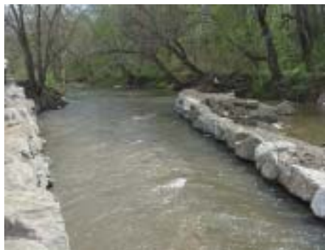
The first arm of the weir begins to have water flow through. Work then began on the second arm. The first stone of the second arm can be seen at right.
