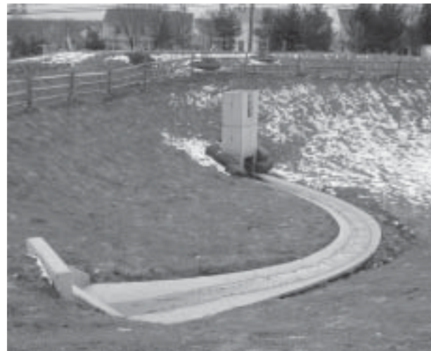
Before: Concrete low flow channel and large orifice at outlet structure provided a quick discharge of stormwater.
