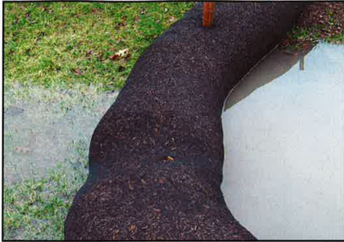
Top: Sediment is filtered out of water as it moves from right to left through the silt sock.
