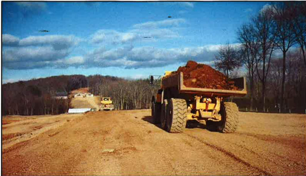
Cut and fill operations on a section of the bypass looking east in November 2010.
