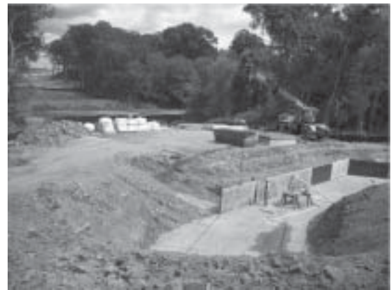
Western abutment foundation under construction in August 2010, for the four-span 202 Parkway bridge over the Neshaminy Creek. Super silt fence has been installed on both sides of the Neshaminy along with "jersey barriers" and a sand bag cofferdam.
