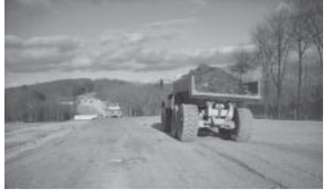
Cut and fill operations on a section of 721 looking east in November 2010. Quail Drive arch culvert can be seen in the center of the photograph.
