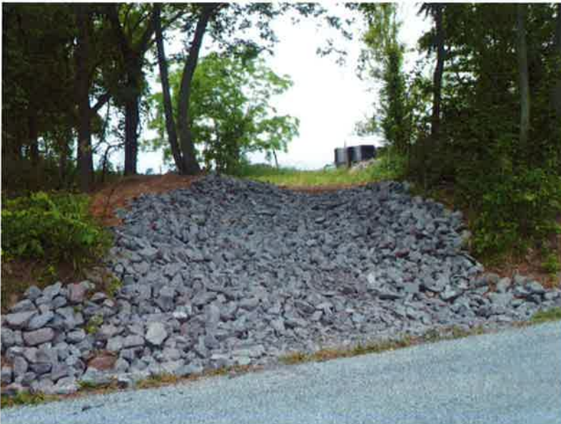
This rock outlet was installed as part of a field diversion project
